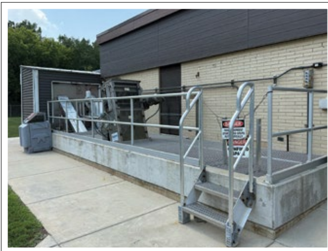
Headworks with new MS2 Bar Screen
