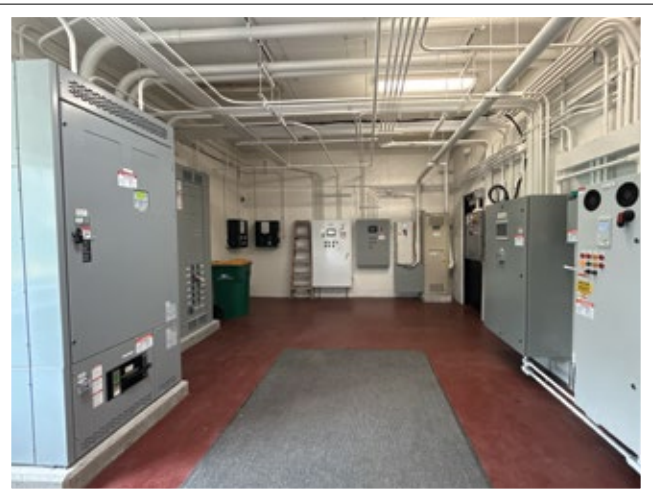
New Control Building Electrical Room
