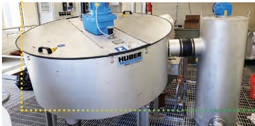
The Huber S-Disc thickener from Energetics, which provides 4% TS to the aerobic/anoxic digester.
