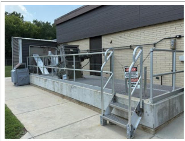
Headworks with new MS2 Bar Screen
