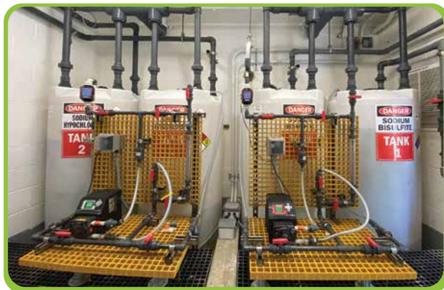
Disinfection Chemical Storage and Feed
