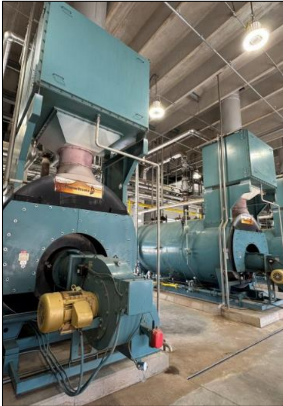
Indirect Hot Water Boilers Typical at WWTPs
